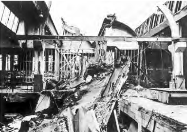
BOMB DAMAGE AT THE MAIN PLANT
