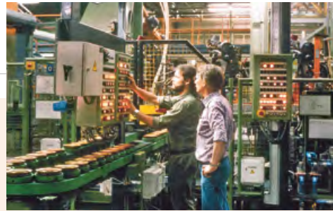
STAFF AT THE CONTROL CONSOLE IN SHED 54
