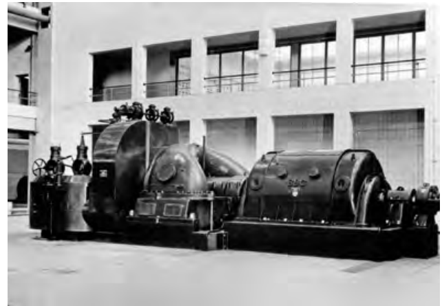
TURBINE SET IN THE POWER PLANT
